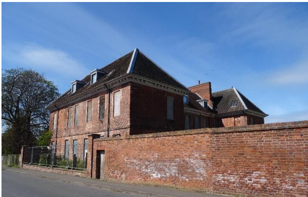
Fig. 22 Ollerton Hall is currently vacant and in a poor condition
